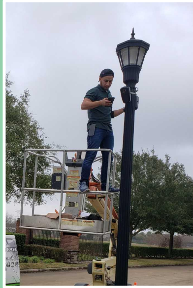
Electric & Existing Pole
