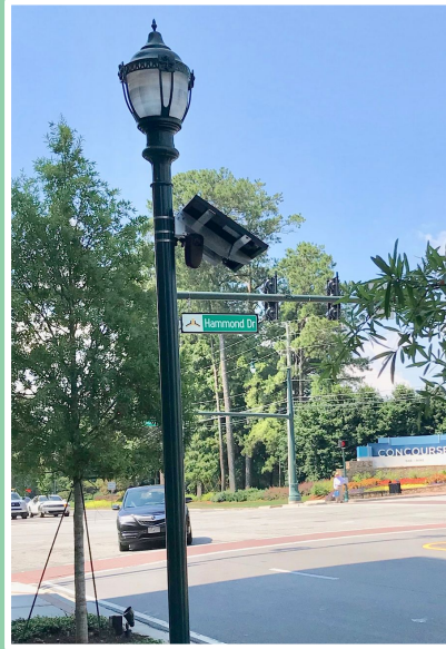
Solar & Existing Pole
